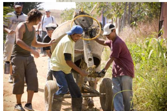
Volunteers and locals work together to provide villagers with concrete floors in their homes.
